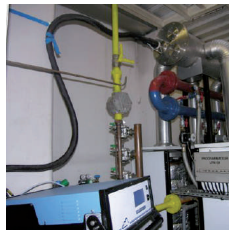
MONITORING OF COMBUSTION GASES ON INDUSTRIAL FURNACE
