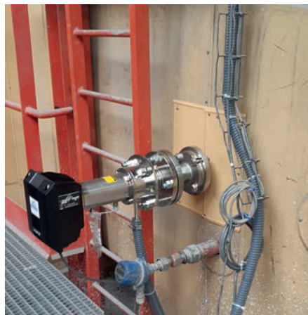
CROSS DUCT, INLINE COMBUSTION MONITORING
